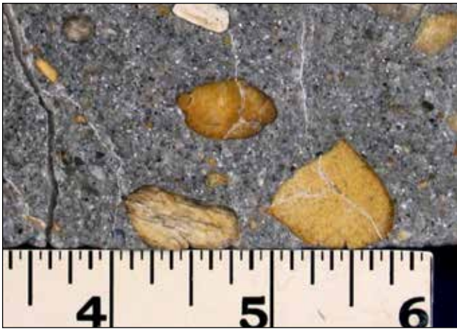
Figure 2: Alkali-silica reaction (ASR) causes certain siliceous aggregates to react with alkalis in concrete to form a gel that swells as it absorbs water from the surrounding cement paste or the environment. These gels can induce enough expansive pressure to damage concrete and leave contractors with no choice but demolition.
