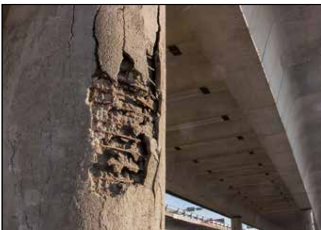
Figure 3: Rebar within concrete corrodes over time, a process that can be accelerated by the ingress of chlorides from deicing salts or ocean spray.
